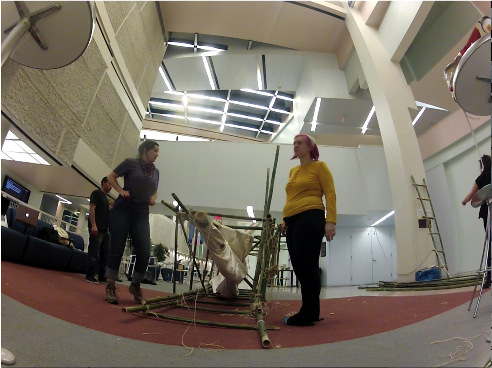
Preparing to raise the scaffold. Click image for video (video credit: Ben Ashworth)
